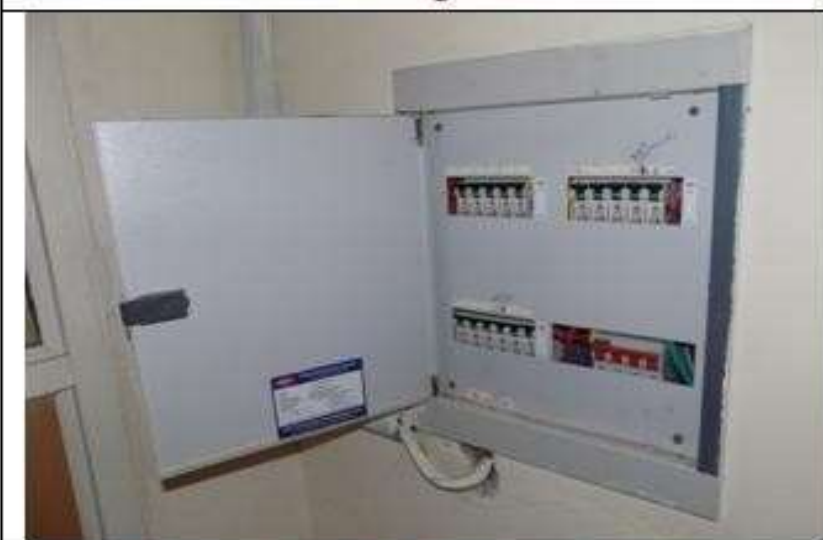
Miniature Circuit Breaker's (MCB's).
