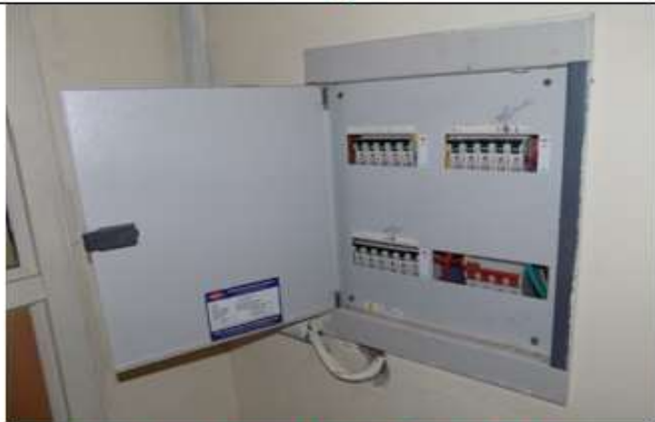
Miniature Circuit Breaker's (MCB's).
